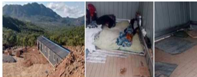
Pictorial Evidence 7: Ming Chang Sino Africa Substandard Accommodation for Staff Source: https://cite.org.zw/chinese-firm-embroiled-in-mine-dispute/
