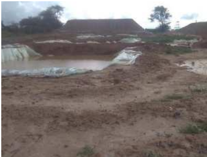
Pictorial Evidence 6: Unprotected Tanks at Dore Green Custom Milling
